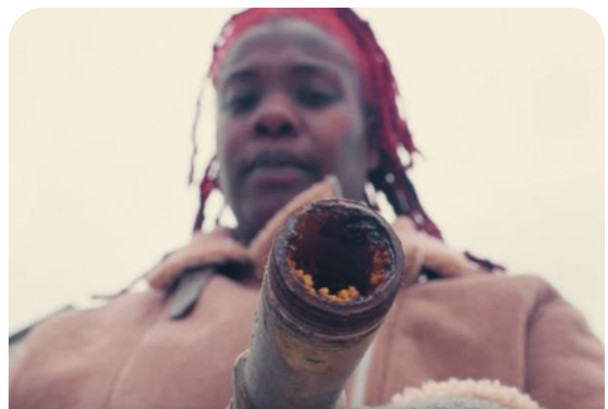
500,000 children in the U.S. are currently exposed to dangerous lead levels, including from pipes like this.
